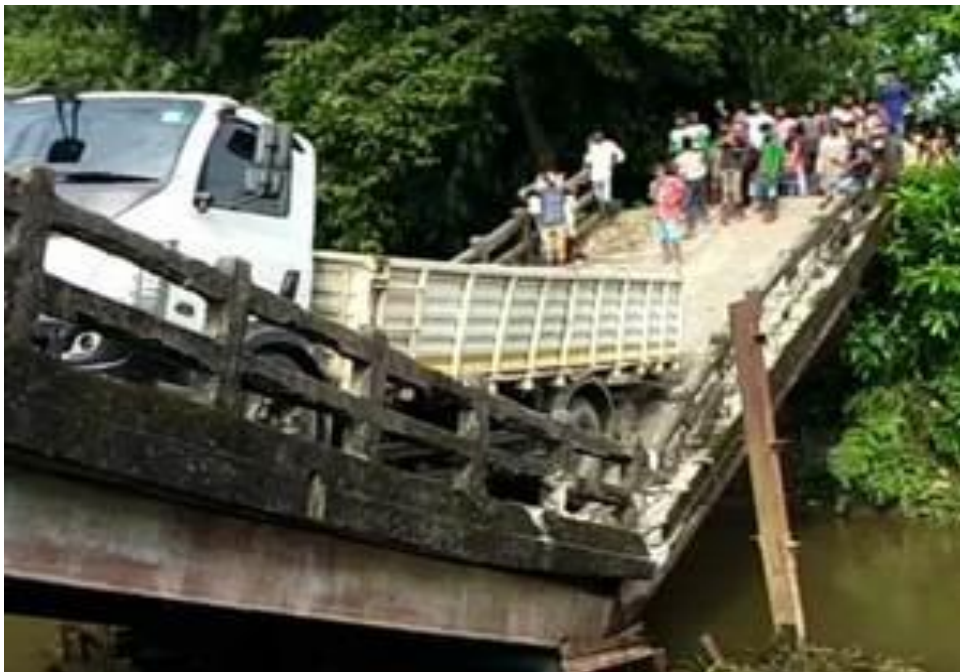
Figure 2 Silguri bridge collapse in 2018
