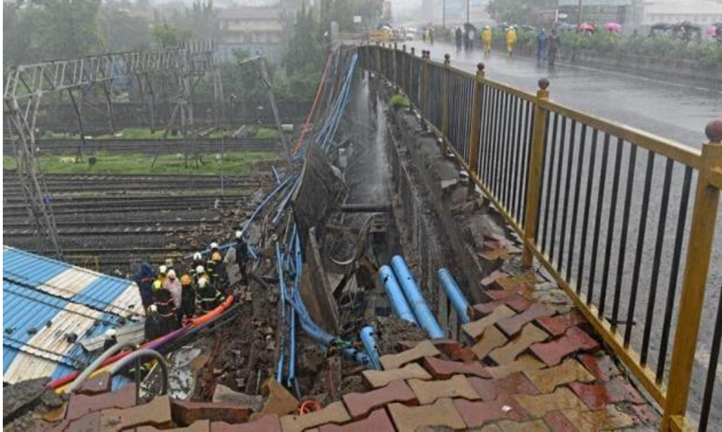
Figure 1 Andheri pedestrian bridge collapse in 2018
